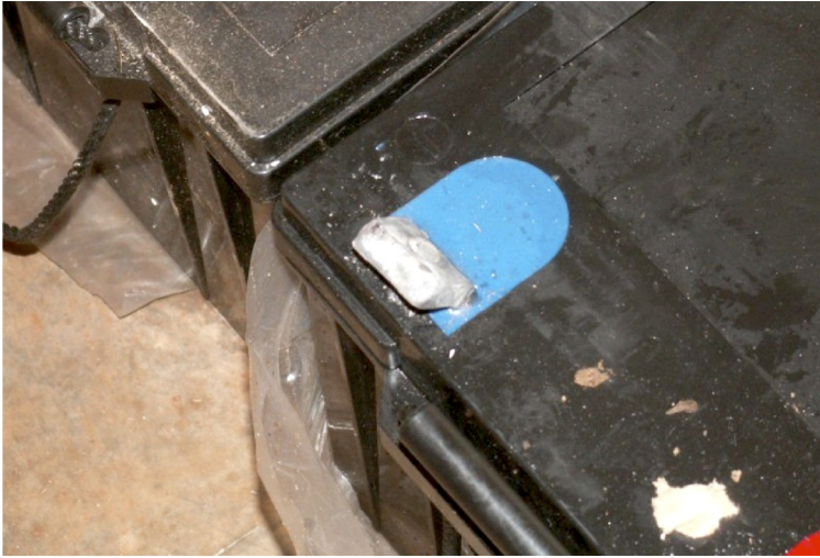
Figure OGP 2: A 200 Ah lead-acid battery. The negative terminal was broken due to weight on the terminals during transportation.
