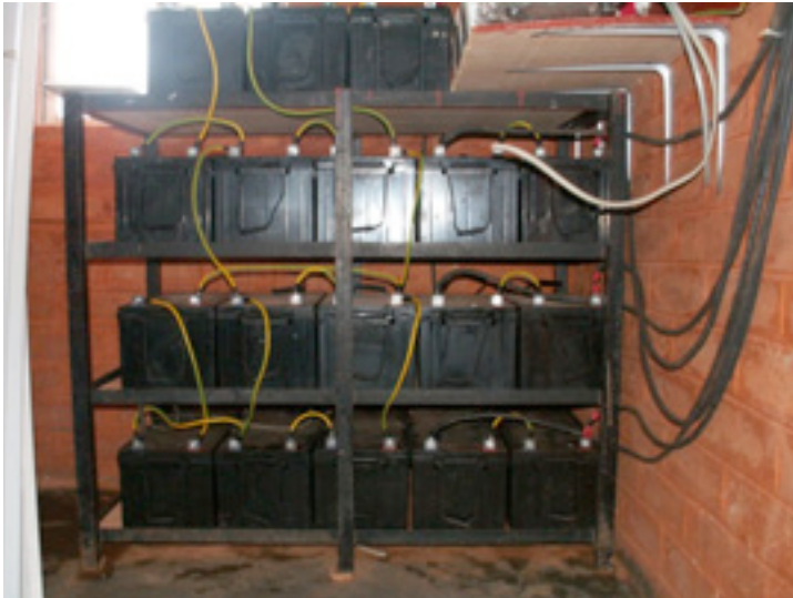
Figure 7.9: A battery bank of 3600 Ah, currents reach levels of 45 A during charging
